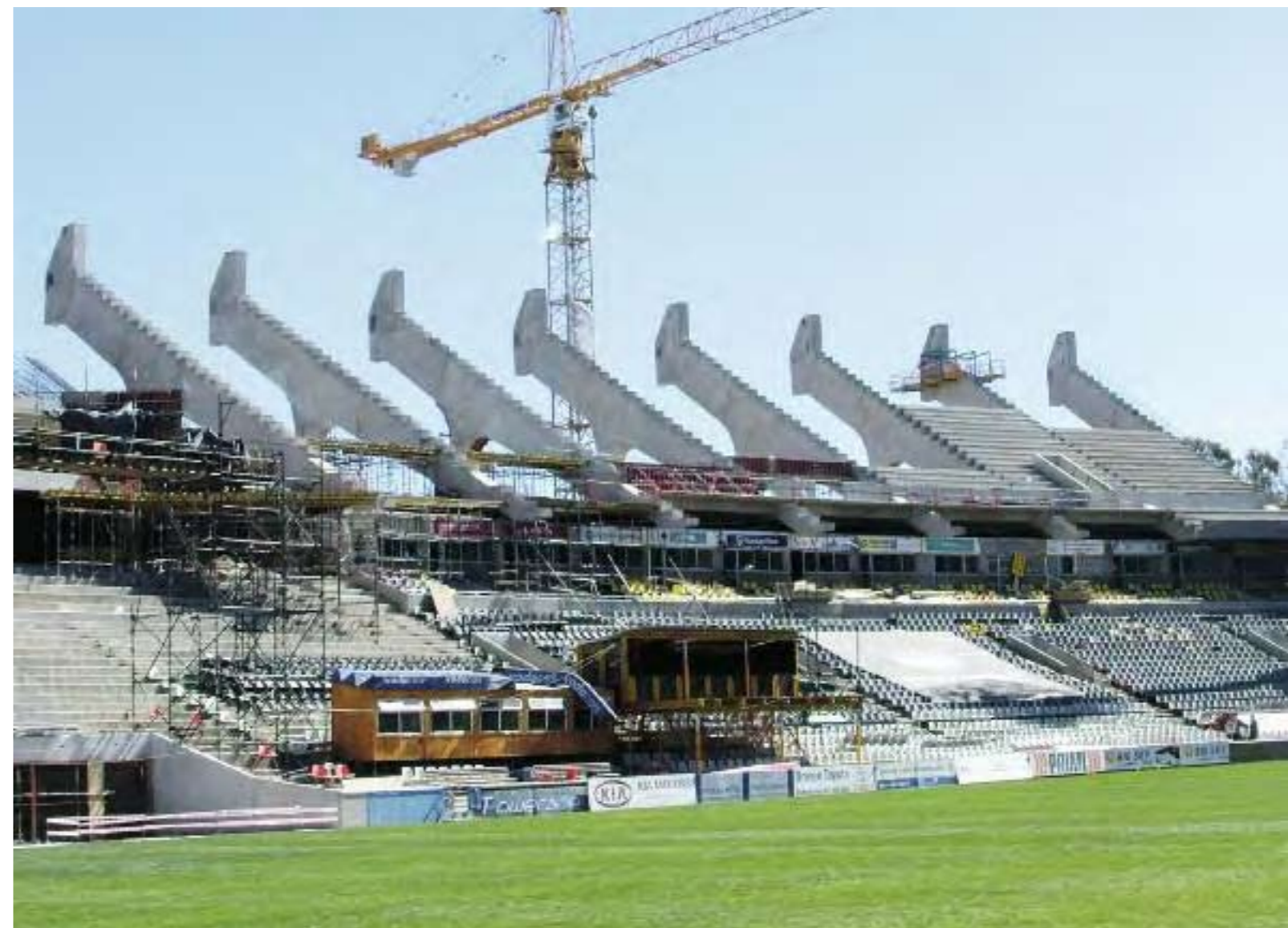
The construction site of the Free State Stadium, made in Lafarge ready-mix concrete, in Bloemfontein, South Africa.
